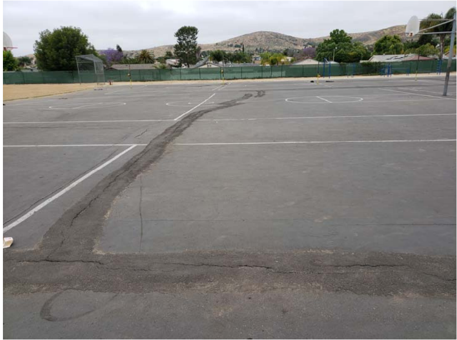
Photograph 3: View of hardcourt play area looking west. Previously patched cracks reopening.
